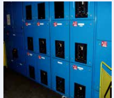
Obsolete Merlin Gerin Selpact ACBs
